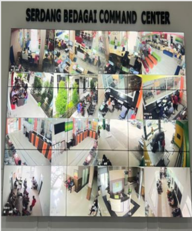
Monitor CCTV Kantor
